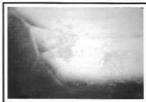
Irregular surface coloration
